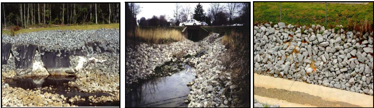
Figure 4. Rock riprap may be a permanent material but this does not mean it will provide the appropriate level of erosion control. Another concern is the potential for piping of soil from between and/or through rock riprap (far right image).
