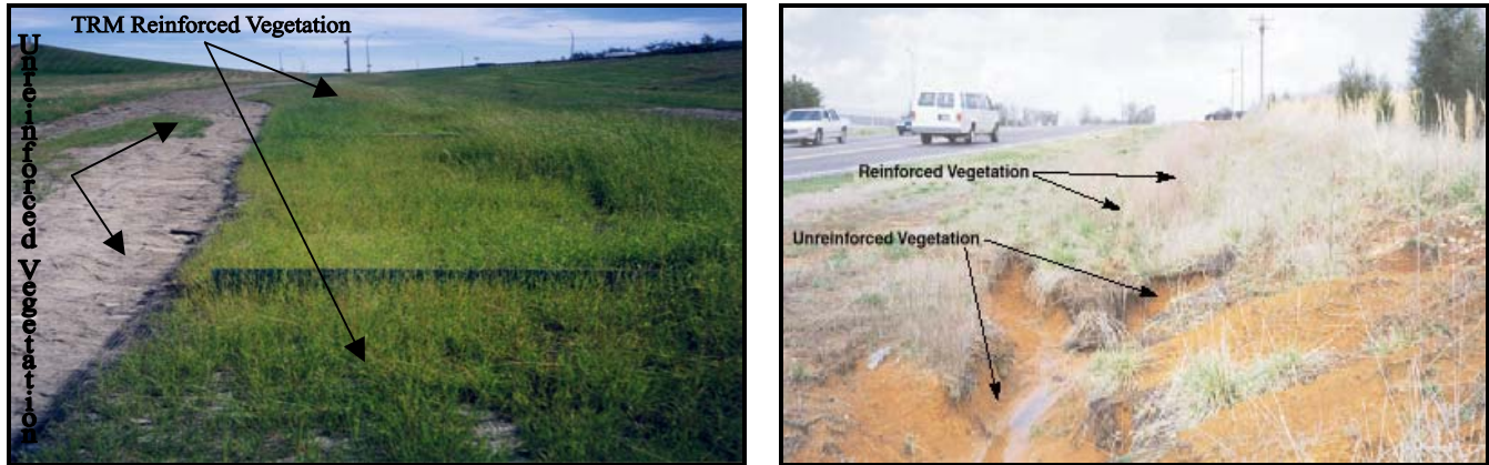
Figure 2. Where the turf reinforcement mattings stop erosion begins. The removal of vegetation and extensive erosion occurred in portions of the same channels where TRMs were not installed . However, those portions of the channel protected by vegetation reinforced with TRMs resulted in exceptional erosion control and turf reinforcement.
